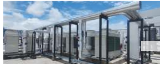
Modular chiller installation for Firmenich Aromatics
