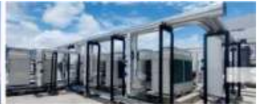
Modular chiller installation for Finerich Aromatics
